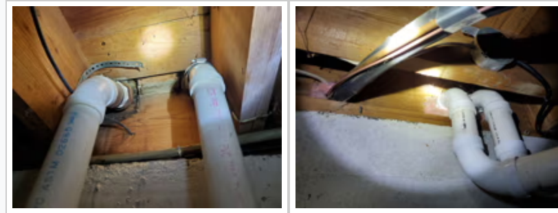
Air Leaks at Penetrations
