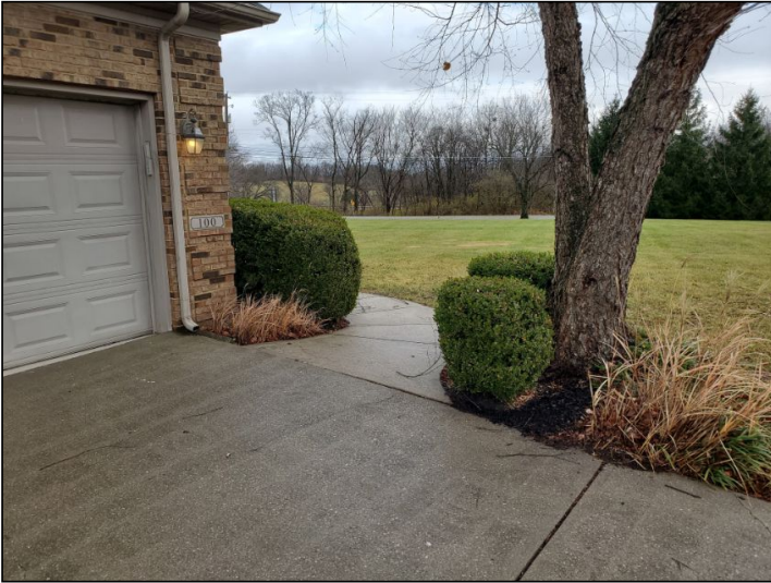
Tree causing concrete to heave
