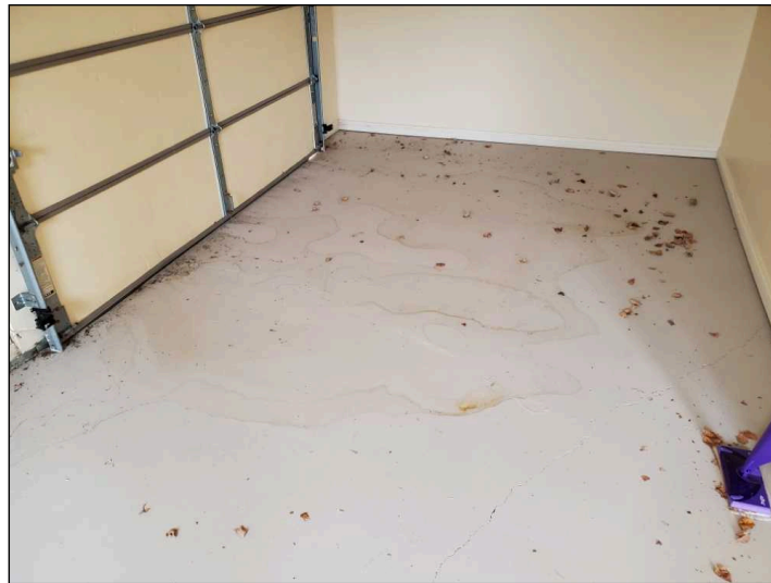
Water entering 2 car garage
