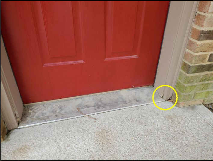
Wood deterioration - Door leading to basement
