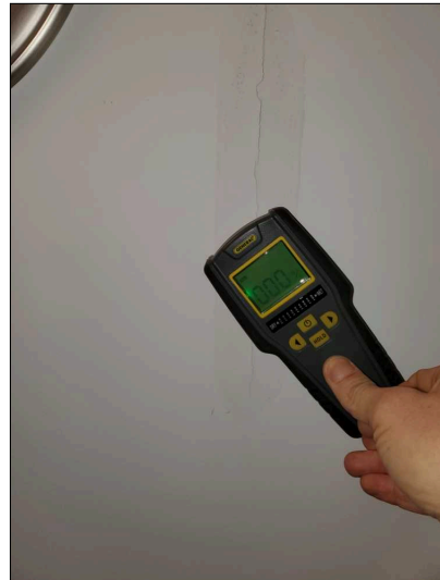
Stain tested dry - Basement ceiling below master bathtub
