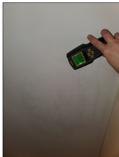
Stain tested dry - Basement hallway
