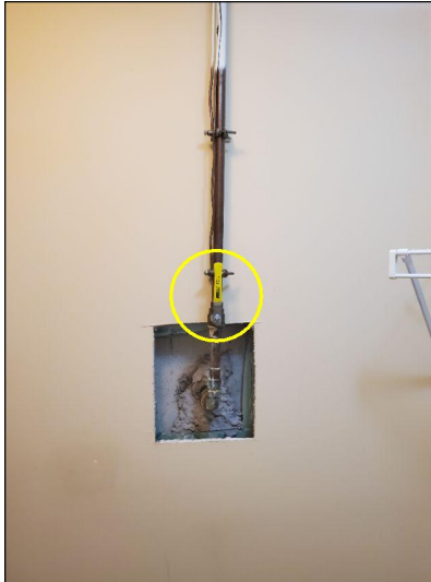
Main Water Shutoff Valve
