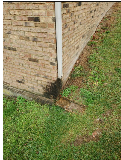
Discharges Near Foundation
