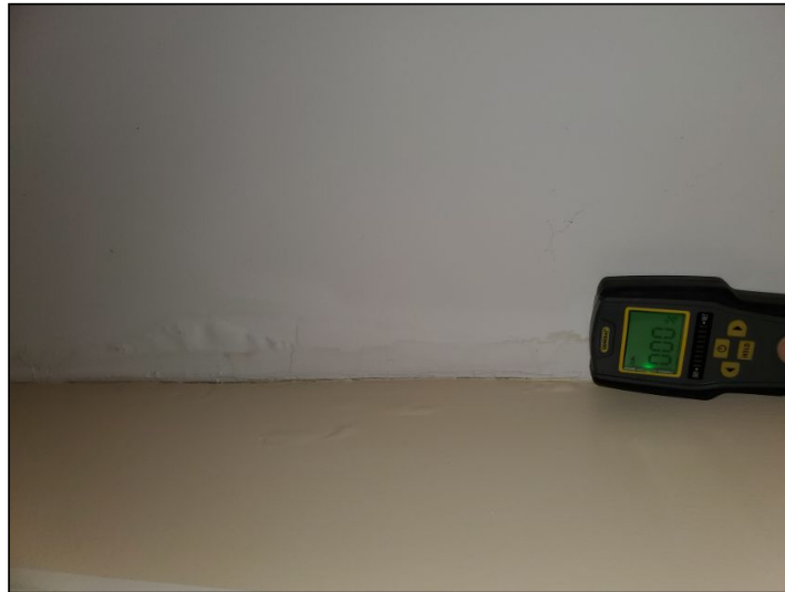
Stain tested dry - Ceiling below exterior kitchen door
