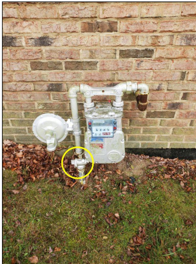
Main Gas Shutoff Valve
