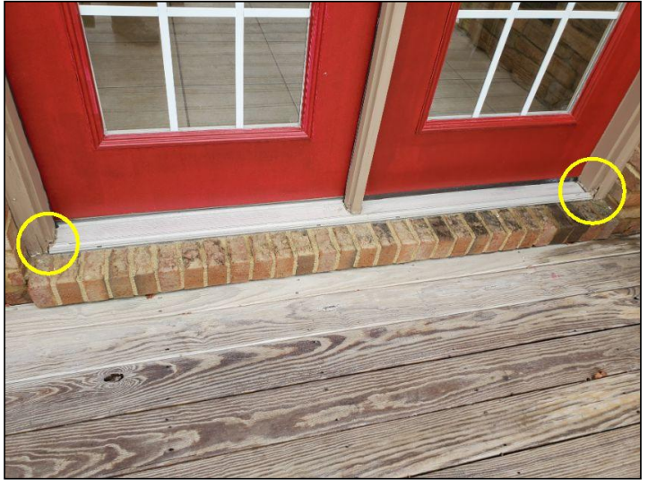
Wood deterioration - Exterior kitchen door
