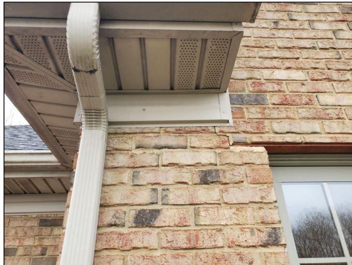
Cracks in brick veneer
