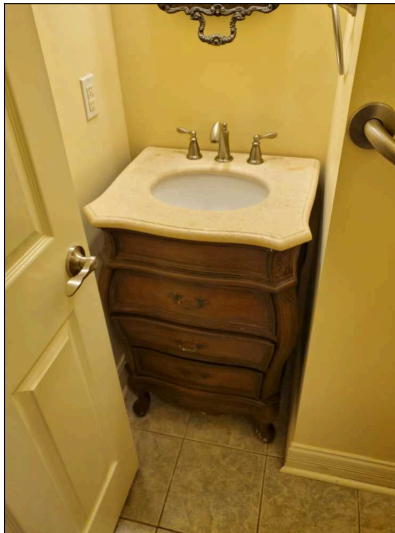
Vanity not secured to wall - 1/2 Bath
