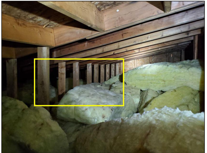
Ceiling joist and rafters bowing due to inadequate support
