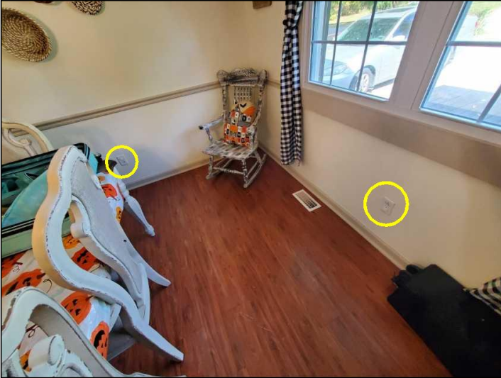
Electrical receptacles not functional - Dining room
