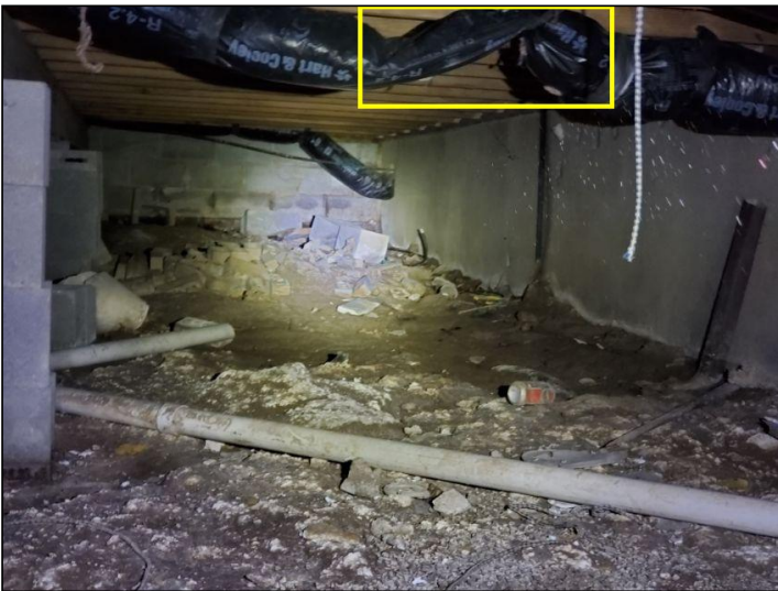
Damaged supply duct in crawlspace below living room
