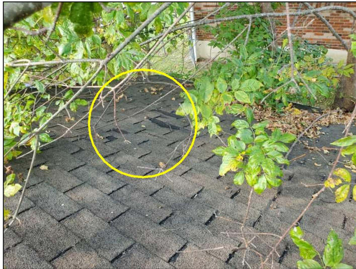
Damaged shingles - Detached garage
