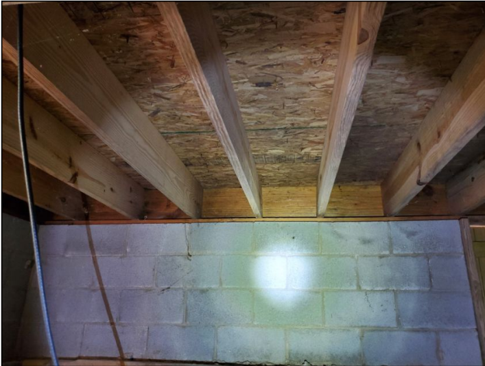
No insulation installed at floor of living room
