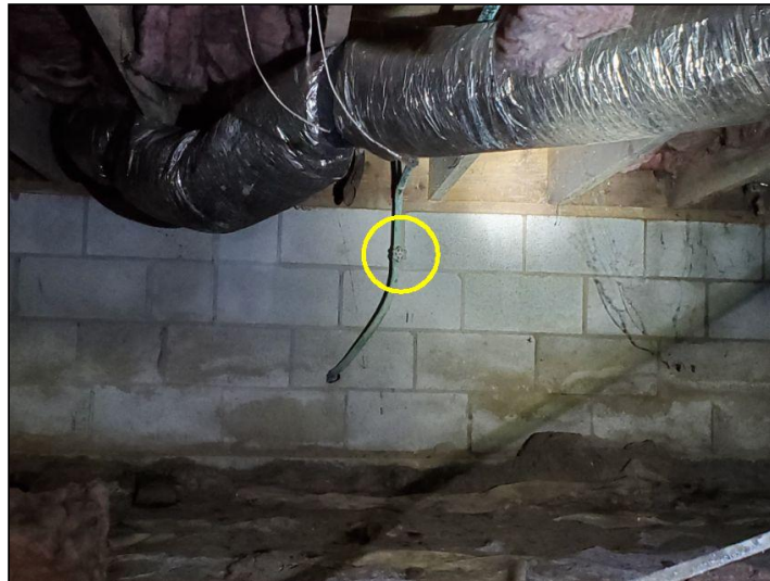
Main water shutoff valve at north side of crawlspace
