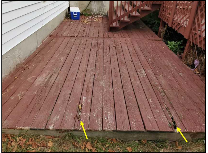
Deck boards deteriorated
