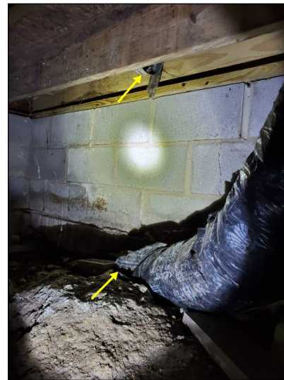
Living room supply duct disconnected
