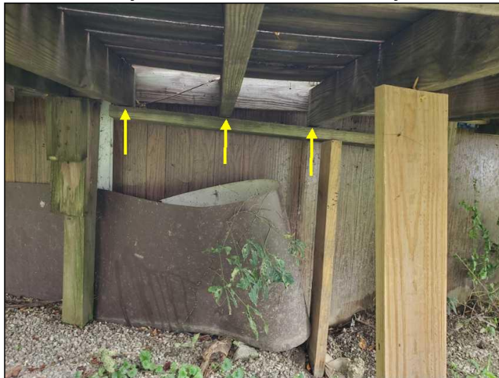
Floor joists not secured to rim joist
