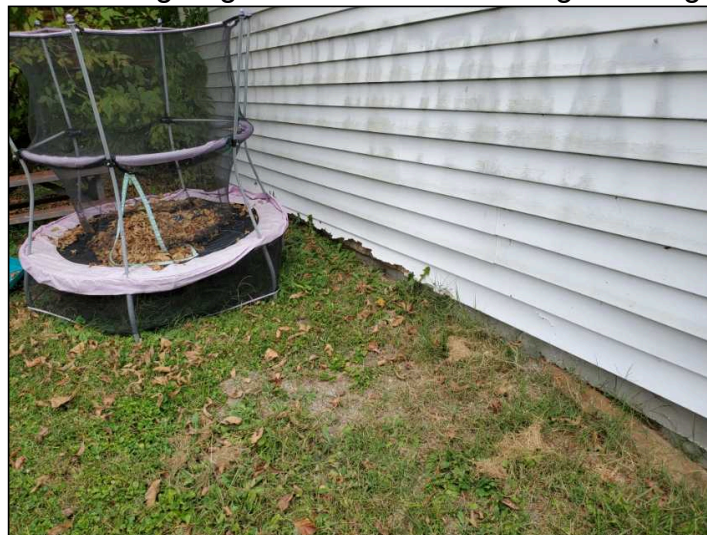
Damaged siding - Detached garage
