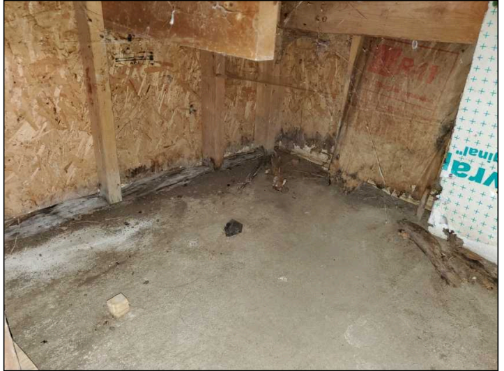
Moisture damage - Detached garage
