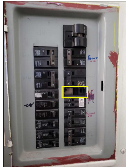
Missing filler plate
