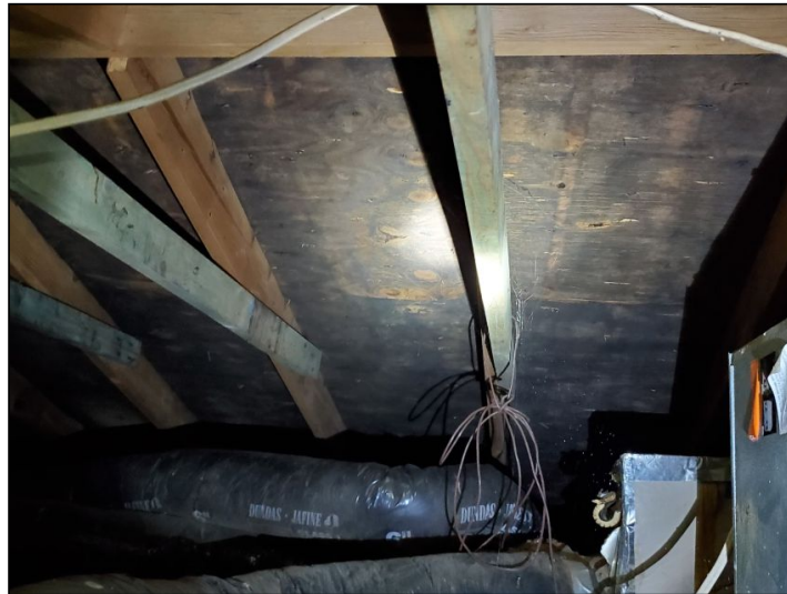
Stains due to lack of ventilation
