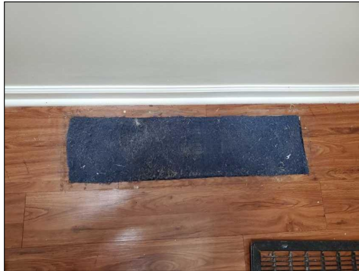
Washable filter inside hallway return grille
