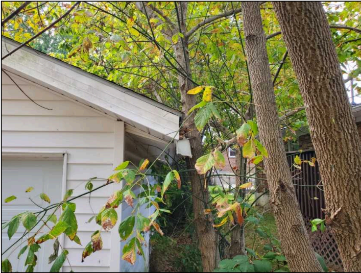
Damaged gutters - Detached garage
