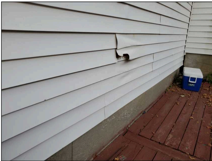
Damaged siding - Detached garage
