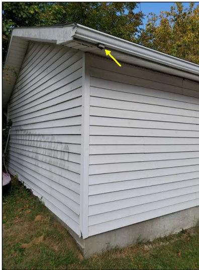
Missing downspout - Detached garage
