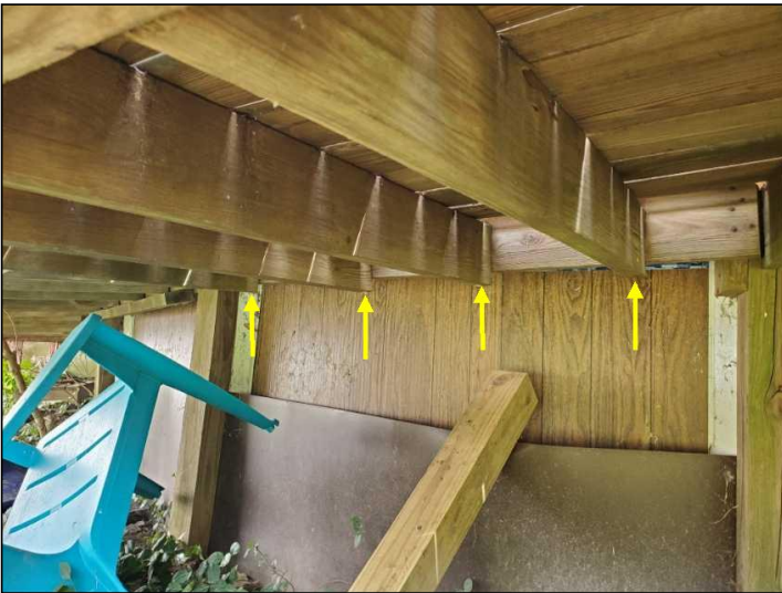
Floor joists not secured to rim joist
