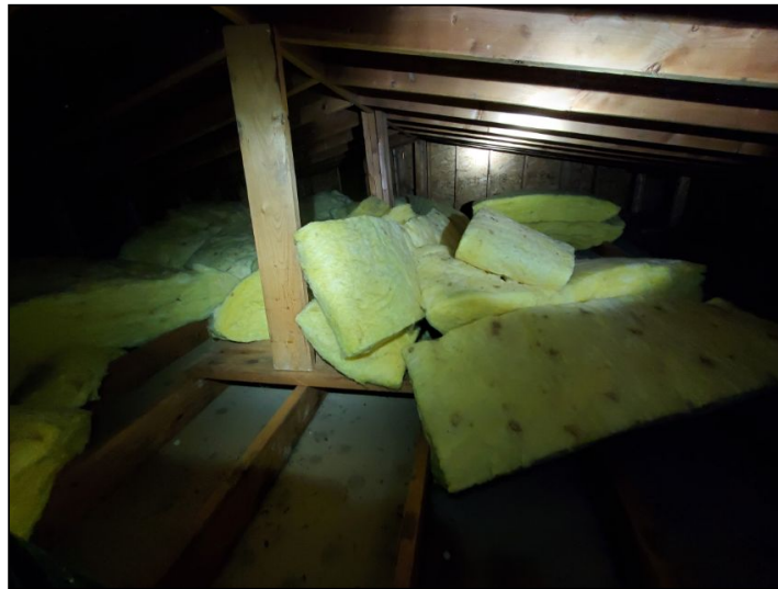
Insulation not in contact with drywall
