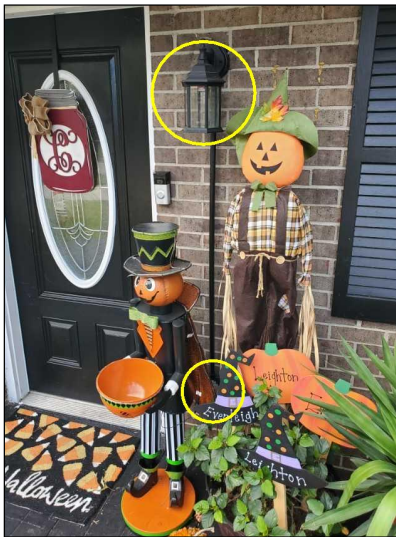
Exterior lights and receptacle not functional
