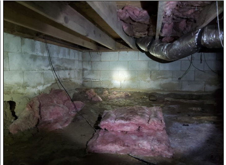
Signs of moisture intrusion at west foundation wall
