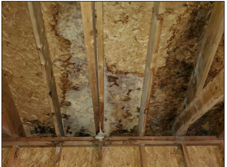
Moisture damage - Detached garage
