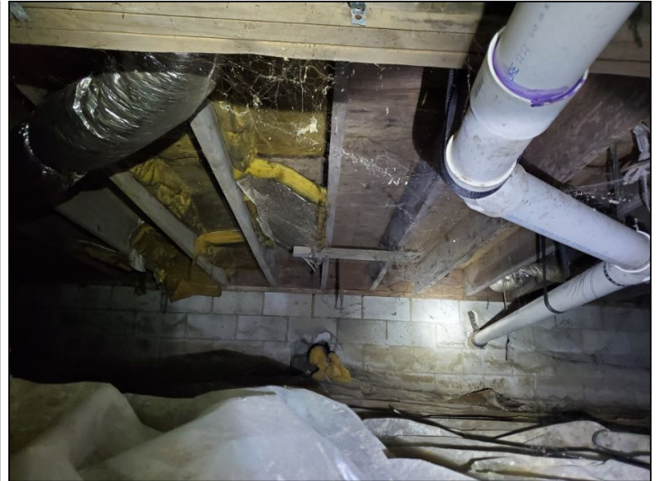
Insulation loose or missing in areas
