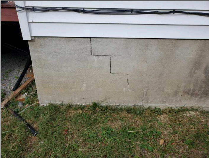
Step crack at foundation wall
