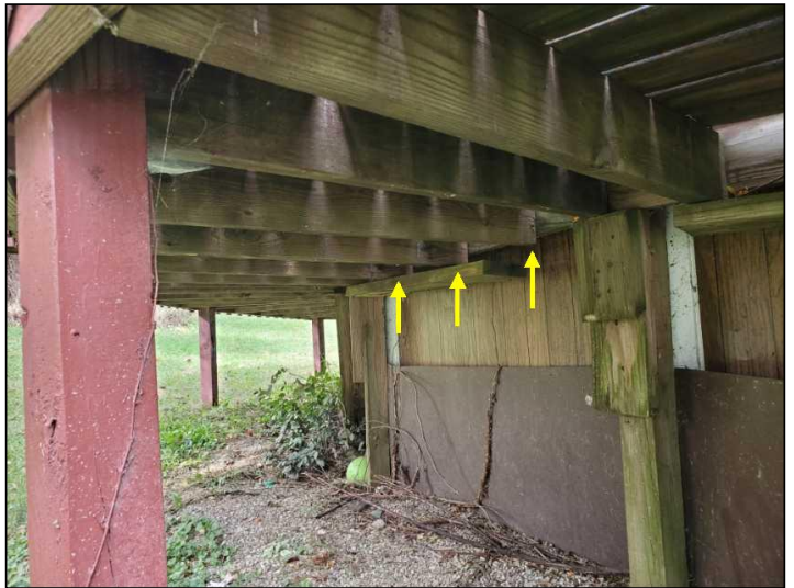
Floor joists not secured to rim joist
