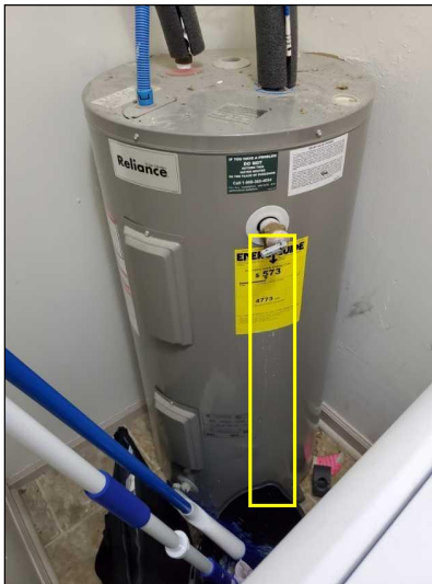
No discharge pipe
