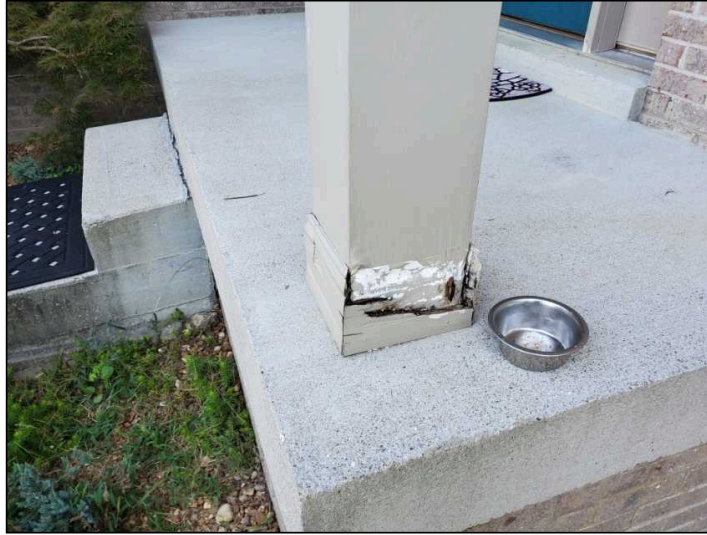
Wood decay - Front porch post
