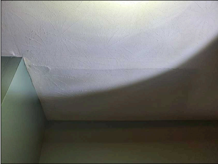
Loose tape - Master bedroom
