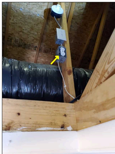
Missing cover plate - Above hallway access door
