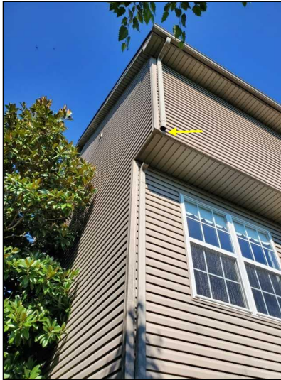
Section of downspout disconnected
