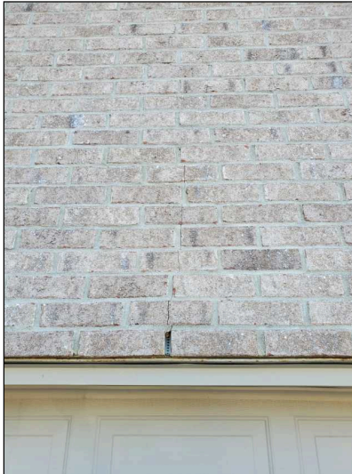
Cracks in the brick veneer - Above garage door
