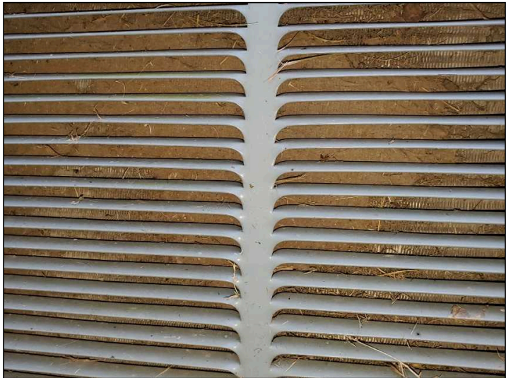
Recommend cleaning coil
