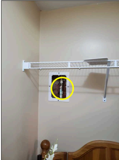
Main Water Shutoff Valve
