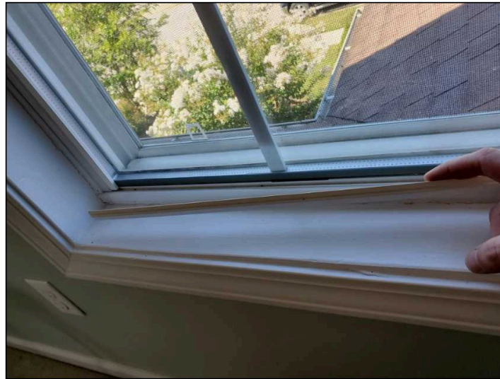
Bottom sash trim damaged - Upstairs bedroom
