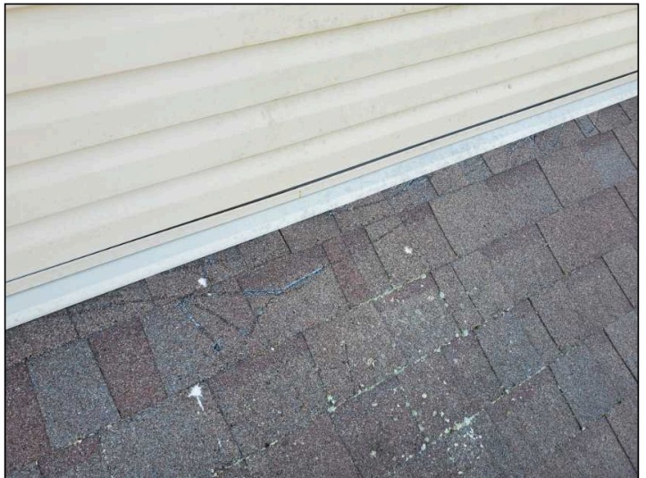
Damaged shingle - Left side of home
