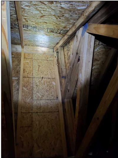
Moisture stains above damaged drywall
