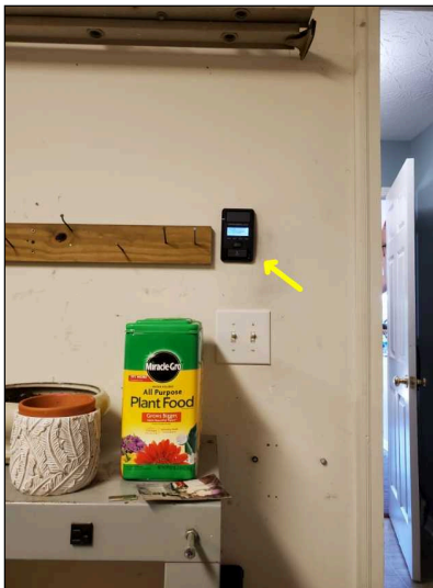
Wall mounted console not functional
